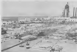
HUNDREDS OF stakes and boards marked the foundation of the structure. CIENTOS DI staca y biga tabata marca fundeshi di e structura.
